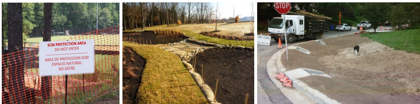
Left: A future bioretention area is protected during construction (adapted from a photo by North Carolina State University Extension); Middle: erosion control measures surround this newly installed bioretention area until construction in the area it is fully completed. (University of Cincinnati's Clermont College, WEF); Right: Inlets are blocked to prevent inflows of stormwater during construction of a bioretention area. (Source: Montgomery County, MD Department of Environmental Protection)
