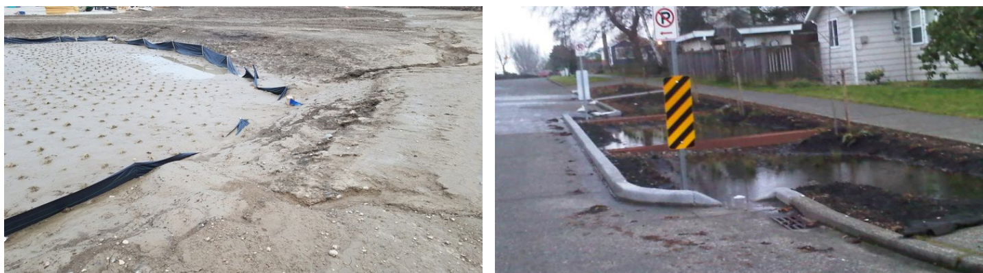
Left: Improper sequencing and poor erosion prevention and sediment control measures destroyed this bioretention area before it could ever start functioning (Source: Cuyahoga Soil & Water Conservation District); Right: Failed bioretention area due to poor land disturbance and construction (Source: City of Ballard, WA)
